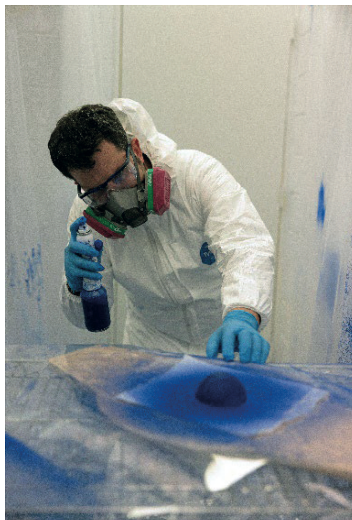
Fig. 2. The author spraying a plaster dome mock-up with a modern mixture of I.K.B.
