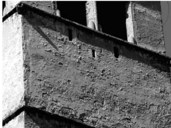
4. Detail of the east façade of the tower: massive plaster formwork on Renaissance plaster due to strong gypsum boarding of surface.
