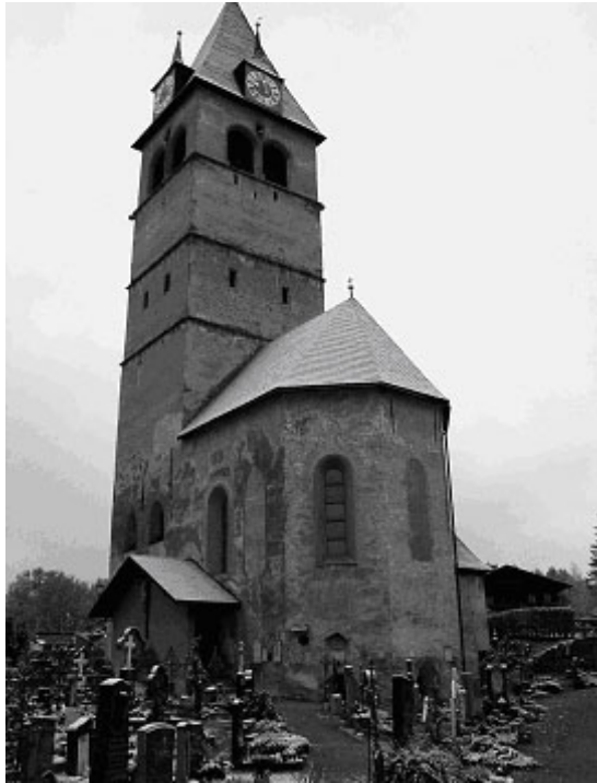
1. Liebfrauenkirche Kitzbühel, Tyrol, Austria. Condition before the restoration.
